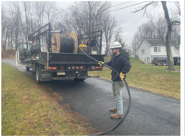
JOB SHADOW: Gettysburg Area High School senior Jayden Cramer pulls secondary wire for a new connection from a lift pole to a meter base in Fairfield, while shadowing a line crew from the Gettysburg District in March. Cramer is the grandson of deceased Adams Electric lineman Charles Kitzmiller, who retired from the co-op in 1994.
